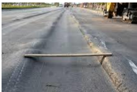
Figure 2.4 Permanent Deformation (Rutting)
