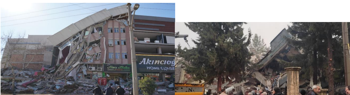
Figure 7. Examples of demolitions and damages in the central district of Adiyaman and Golbasi
