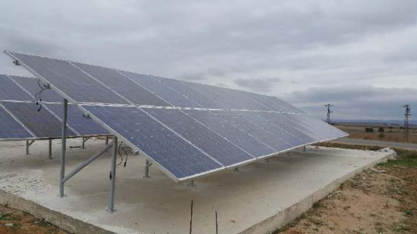
Figure 6. Solar Panel Array
