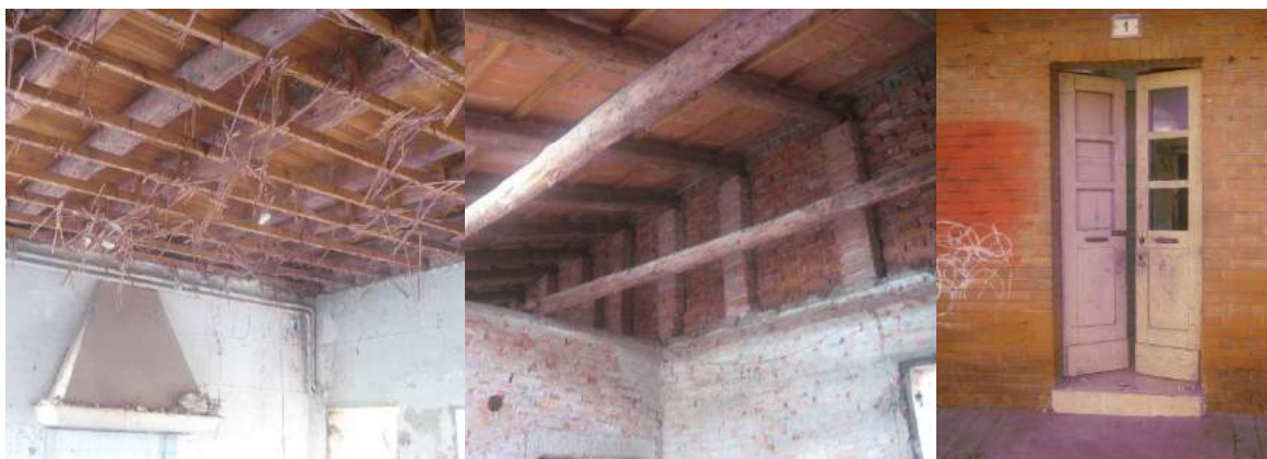
Figures 11, 12, 13. The rural houses that close off the southern side of the new piazza in Vigonza (1937-1938). Details of the original situation: the wooden intermediate floors, the masonry that supports the beams of the single-pitched roof, the doors and windows made of wood and painted white.
